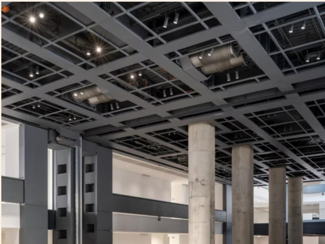
Exposed vents in the ceiling of Fondation Cartier © Martin Argyroglo
